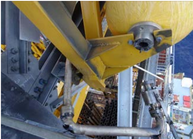
Failed CAPV and Interconnected Pipe
