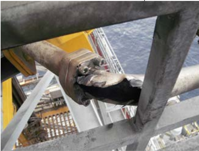
Ruptured Interconnected Pipe
