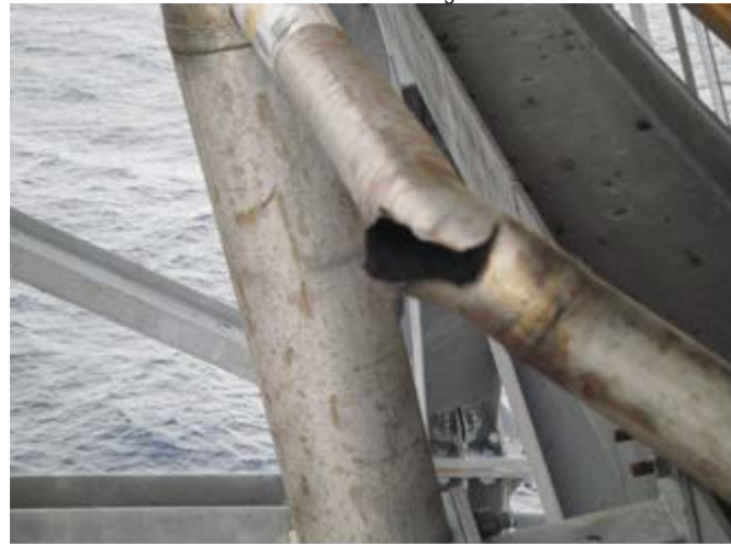
Ruptured Interconnected Pipe
