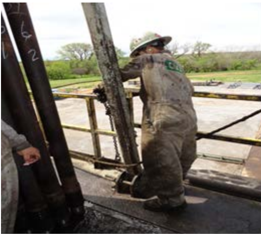
Position of the Injured Employee prior to his fall and the position of the snatch block chain.
